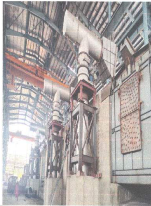
Induction furnace connected with primary hood
