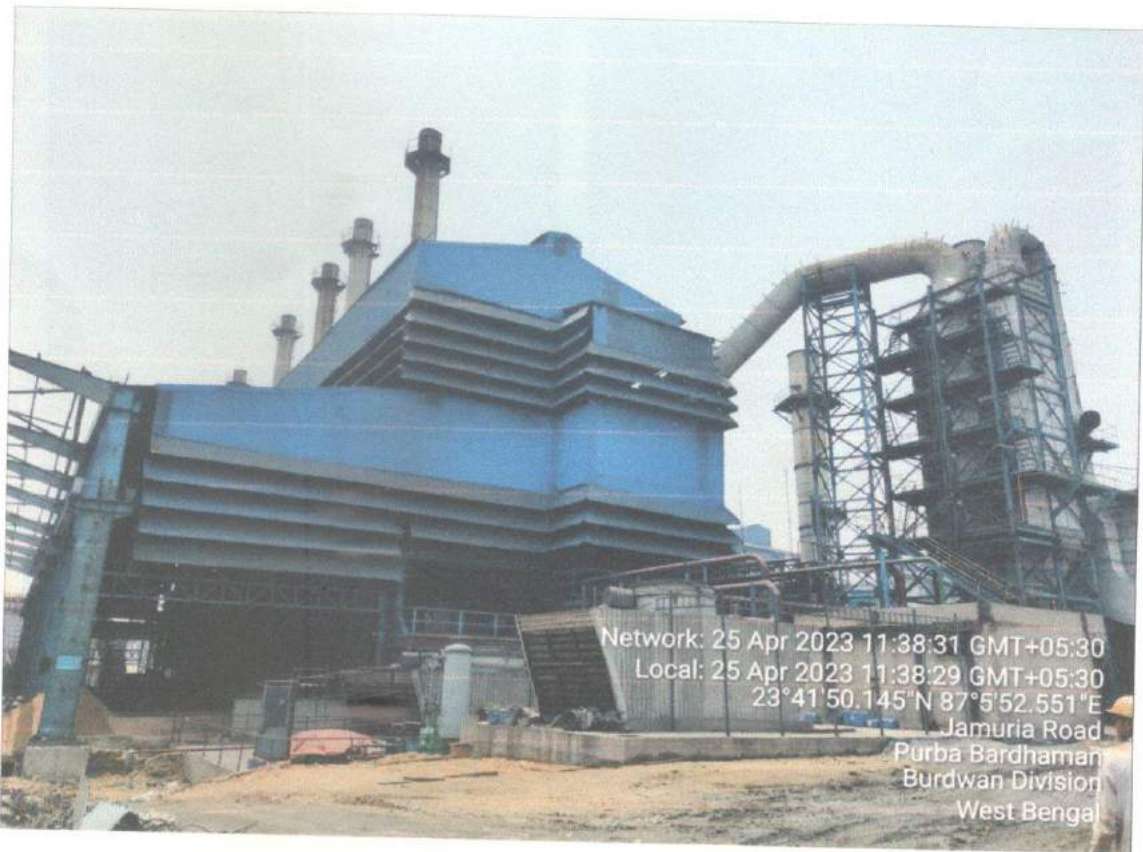
Bag Filter connected with 2x9 MVA SEAF
