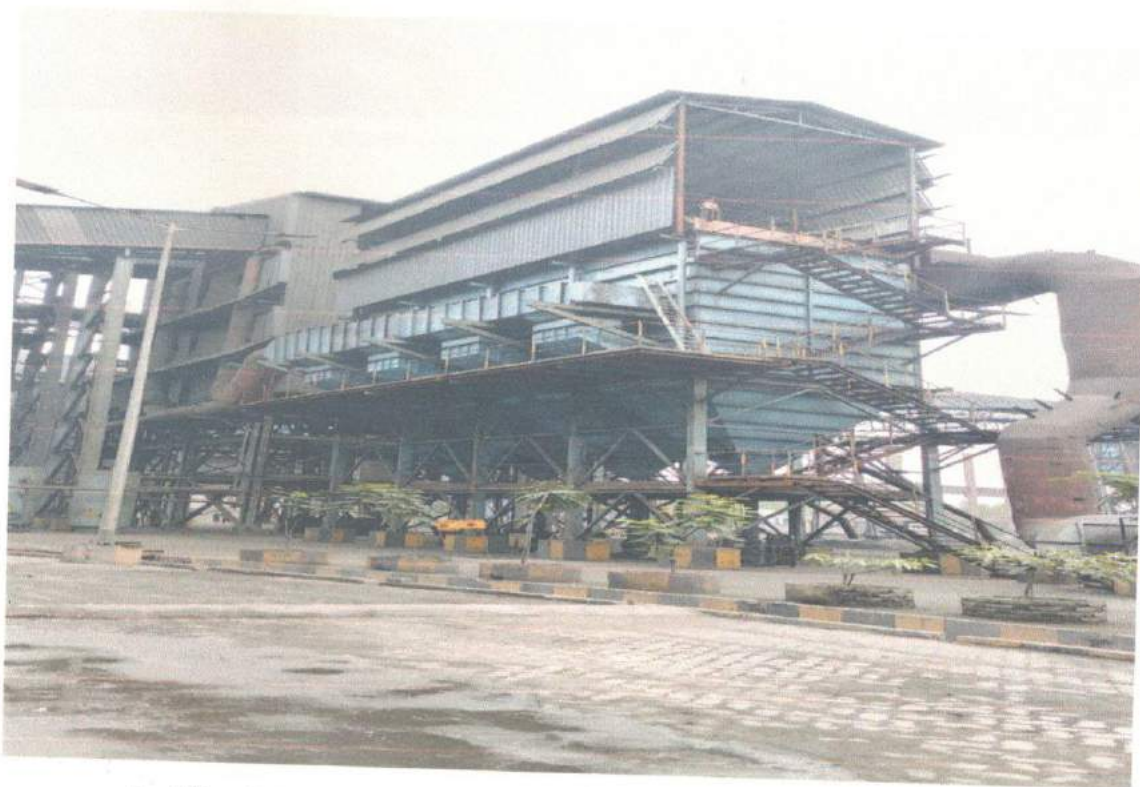
Bag Filter Connected with DRI 300 & 600 TPD (product separation & dispatch)
