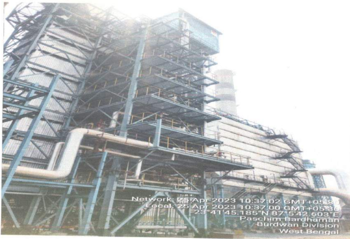
5 field ESP connected with 600 TPD DRI through WHRB
