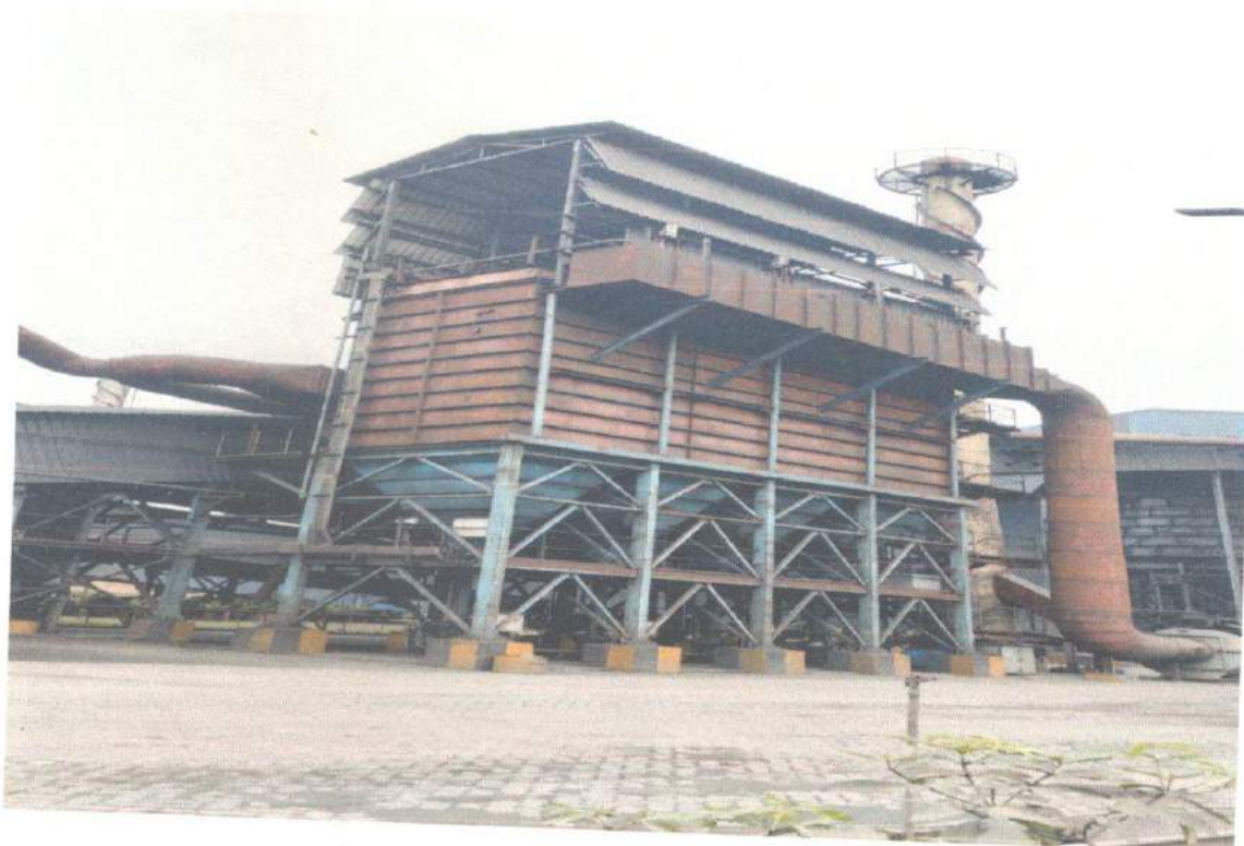
Bag filter connected with CD & I-Bin of 300 TPD DRI
